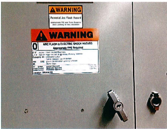
Figure 6: Hole in Arc Flash Barrier.
